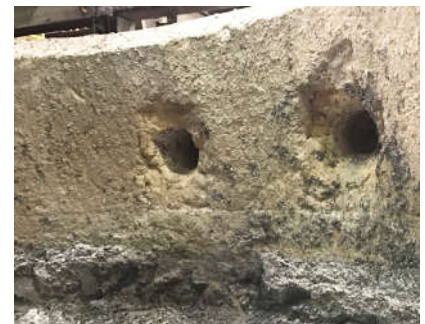
Furnace at current state
